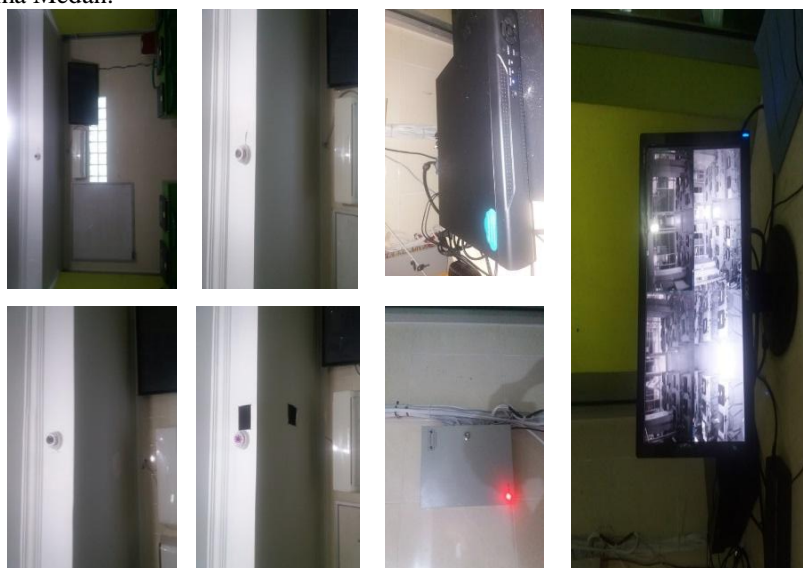
Gambar 5. Instalasi CCTV di Laboratorium STMK Budi Darma
